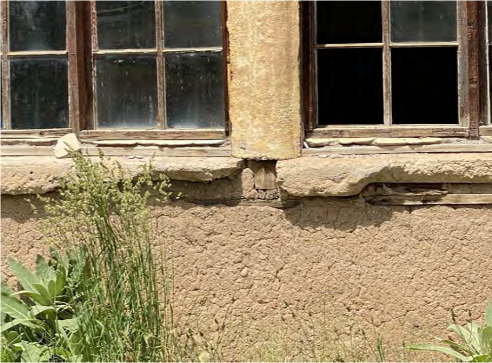
Concrete sills are cracked revealing the wood framing that supports the lintels bearing the wall and roof weight. The point load bears on the adobe wall beneath the window.
